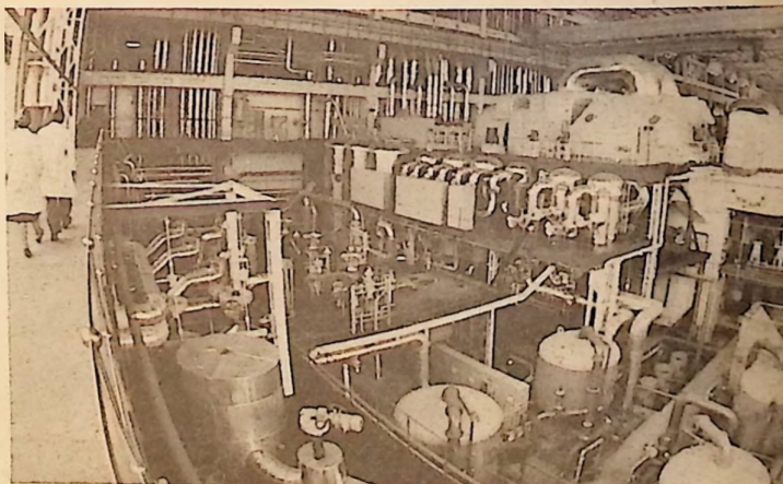
In this gleaming spotless section the atom's power, converted to super-hot steam, roars through turbines that deliver electricity. By-product plutonium is most efficient of all nuclear station fuels.
