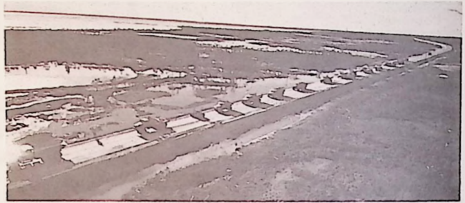
New motor road in very far north (Tyumen) oil region cost 3 million roubles per KM (7 million dollars per mile!). First it was deep-frozen, then covered with insulation (peat), finally surfaced for traffic.
