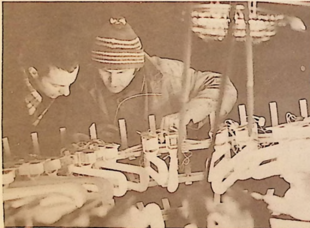
Skilled technicians installing the lights, which are a splendid feature of all subways in Soviet Union.
